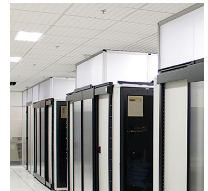
Floor Mounted Hot Aisle Containment
