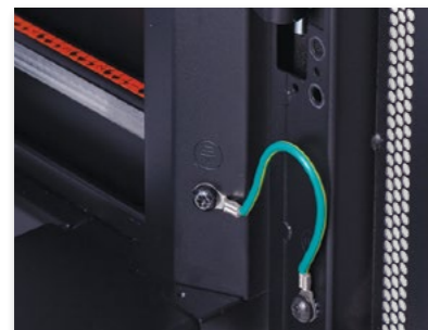
Integrated Electrical Grounding
